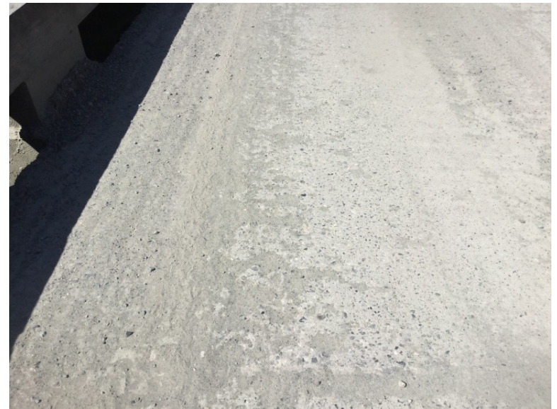
Panels wearing across deck on wheel path
