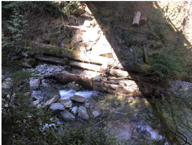
Partial old log crib still in tact at left bank
